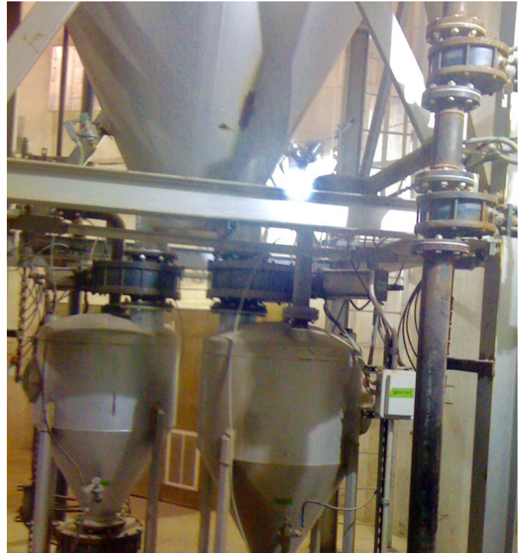
ADM FBC Co-Gen Bed Ash, 300F Vacuum System
