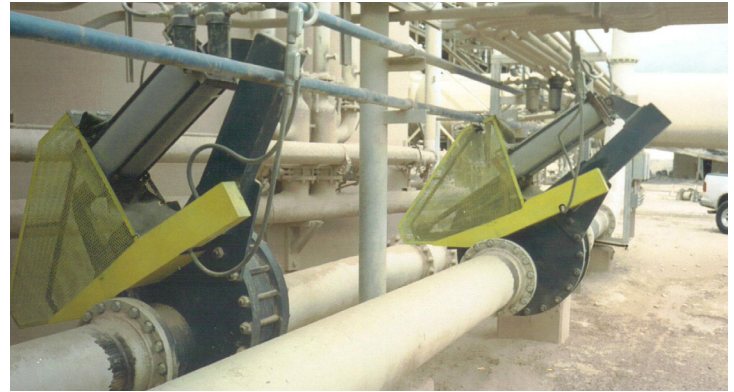
Iron sulfide fines conveying, with Protective Guarding
